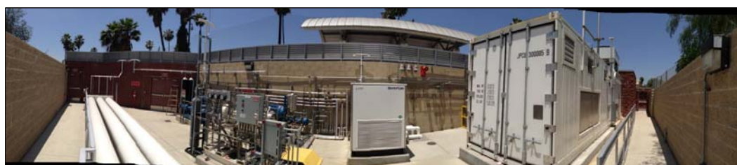
Storage banks (6k psi) Compressors H 2 chiller (-20°C) Electrolyzer with O 2 vent
